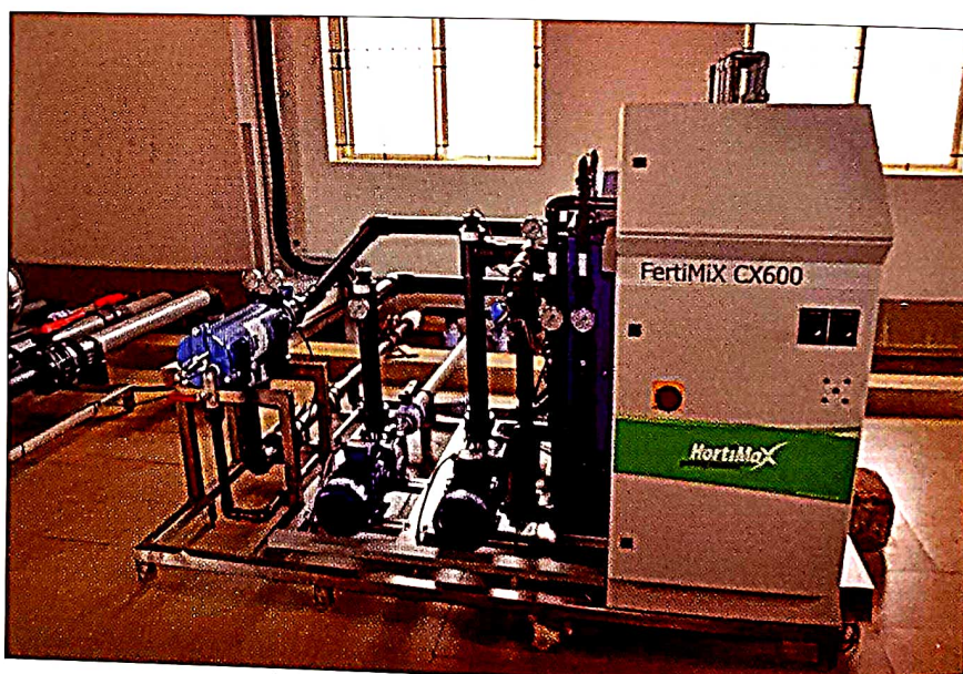
Automated Fertigation System
